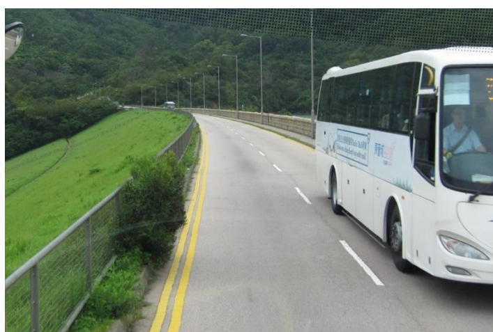
Steep Side Slope of the Dam without a Proper Safety Barrier
