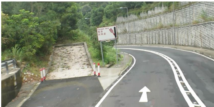
General View of the Arrester Bed for Northbound Traffic: Out-of-control vehicle is likely to overrun the facility and roll down the side slope back onto the road
